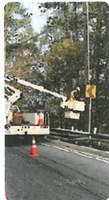
City Foot Traffic Street Electric & existing pole
