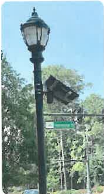
City intersection Solar & existing pole
